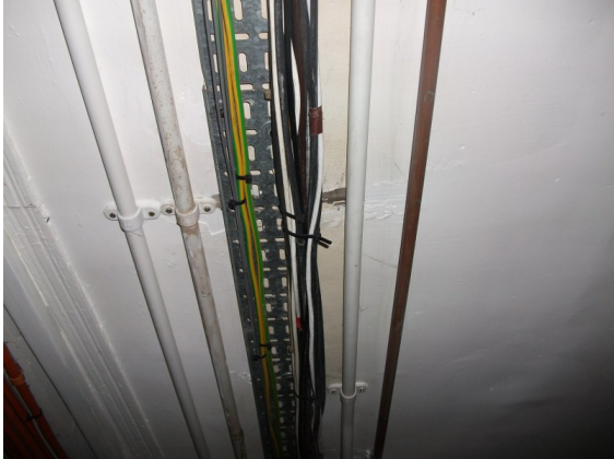
Wiring systems in basement area liable to collapse in the event of a fire.
