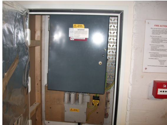
Example of common part services cupboard door fitted with intumescent strips and smoke seals.
