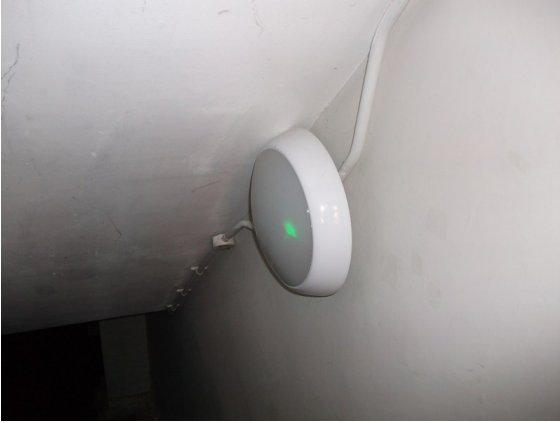
Example of emergency lighting.
