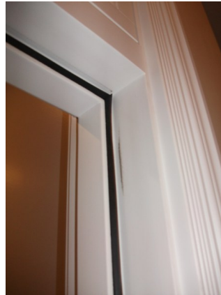
Smoke seal fitted to flat entrance door frame.
