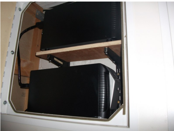
Example of common part services cupboard door fitted with intumescent strips and smoke seals.
