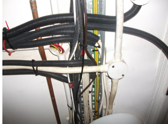
Wiring systems in basement area liable to collapse in the event of a fire.
