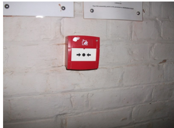
Break glass call point in basement corridors.
