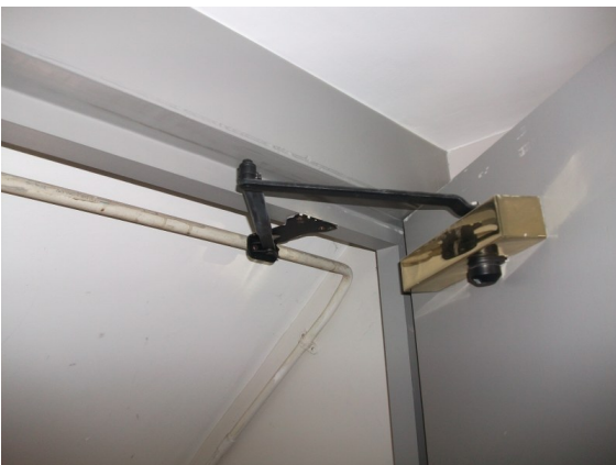
Self-closing mechanism fitted to common part fire doors.
