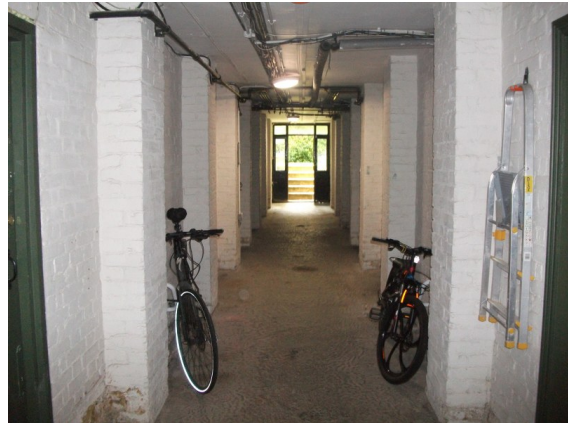
Wires liable to collapse.
