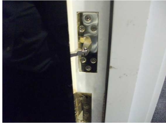
Self-closing mechanism fitted to flat entrance doors.
