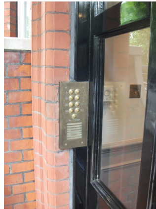
Secure access to all blocks.
