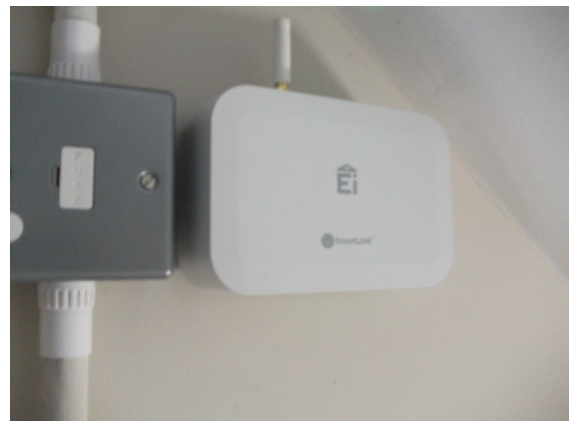
Fire alarm WIFI repeater.
