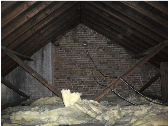
Example of fire separation in loft space.
