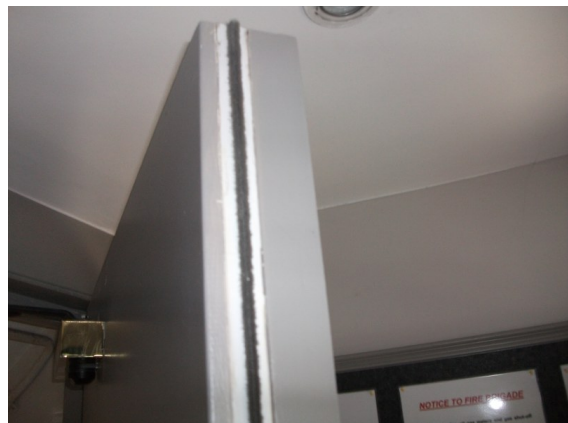
Intumescent strips and smoke seals fitted to common part fire doors.
