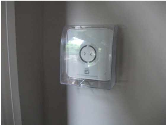
AICO wireless fire alarm system.
