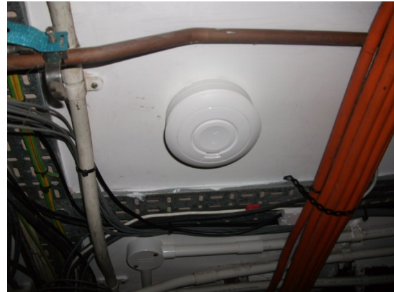
Detection in basement area.
