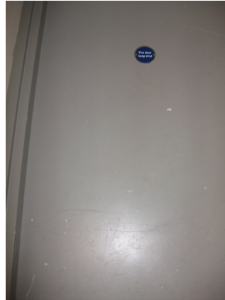
Common part fire door with appropriate signage.
