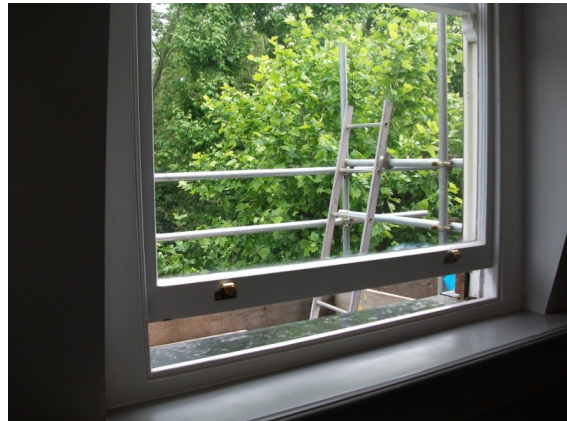
Example of window on second floor and above with restrictors fitted.
