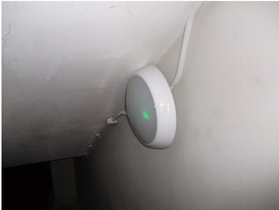
Emergency lighting provided.
